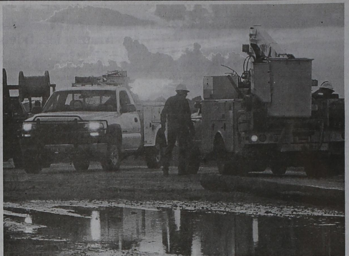
Employees of Lyntegar Electric Coop worked through the night last Saturday and Sunday repairing powerlines toppled by thunder storms that hit the area around Graham Community. The above photo is in front of the home where Mr. and Mrs. E.M. Norman used to live (the old Norman home). Xcel Energy out of Amarillo was also dispatched to handle powerline repairs in the area. (Staff photo by Tim Burnett)
