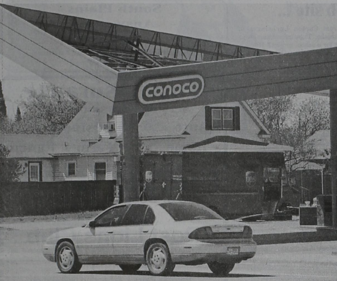
The local Wes-T-Go Conoco station suffered major damage to the gas pump over-hang as a result of the strong winds that visited Post last week. Repairs were completed by Saturday for weekend traffic. (Staff photo by Tim Burnett)
