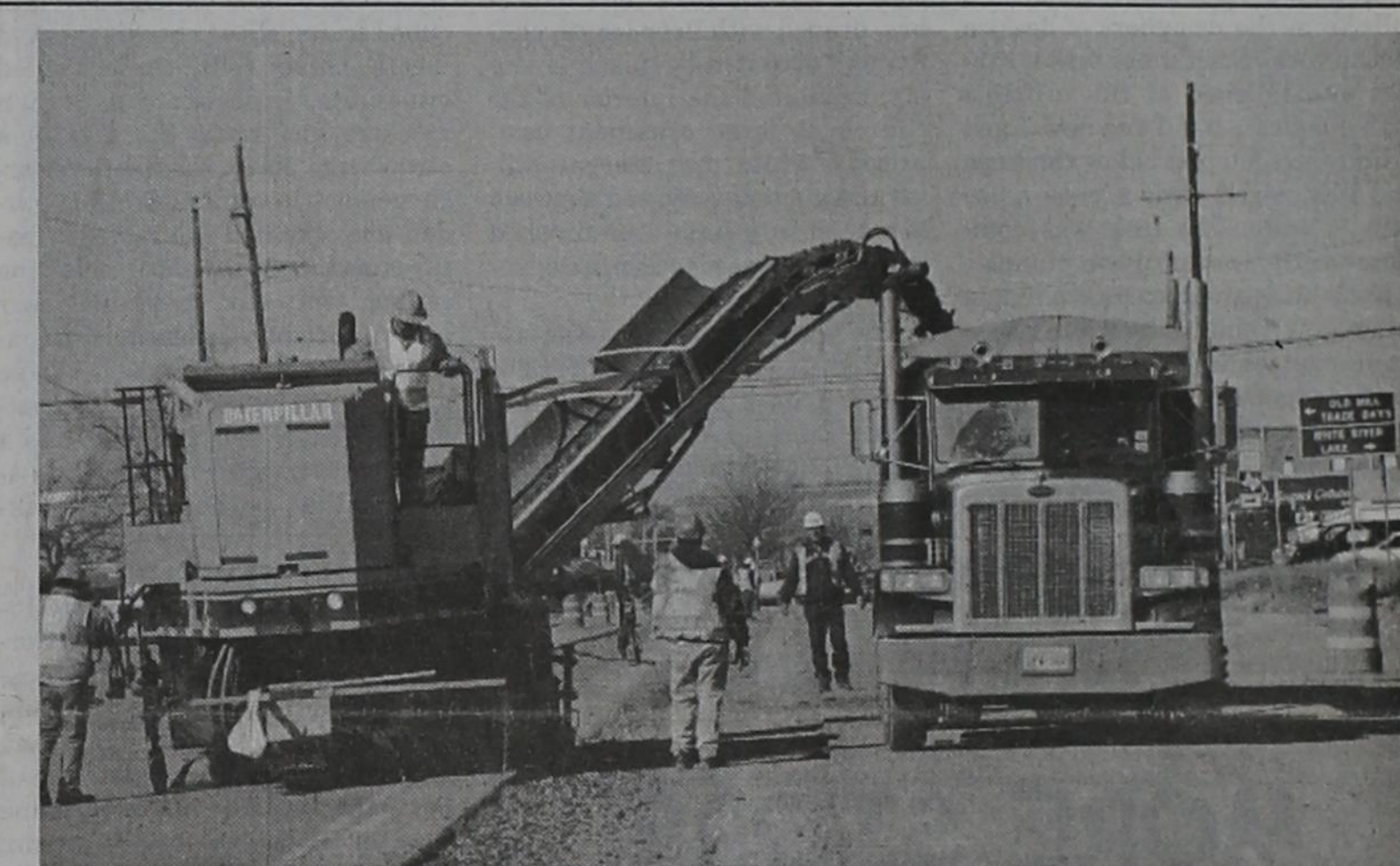
Traffic along U.S. Hwy 380 east is being disrupted while reconstructive work is completed on the roadway from the railroad tracks east to the county line. (Photo by Tim Burnett)
