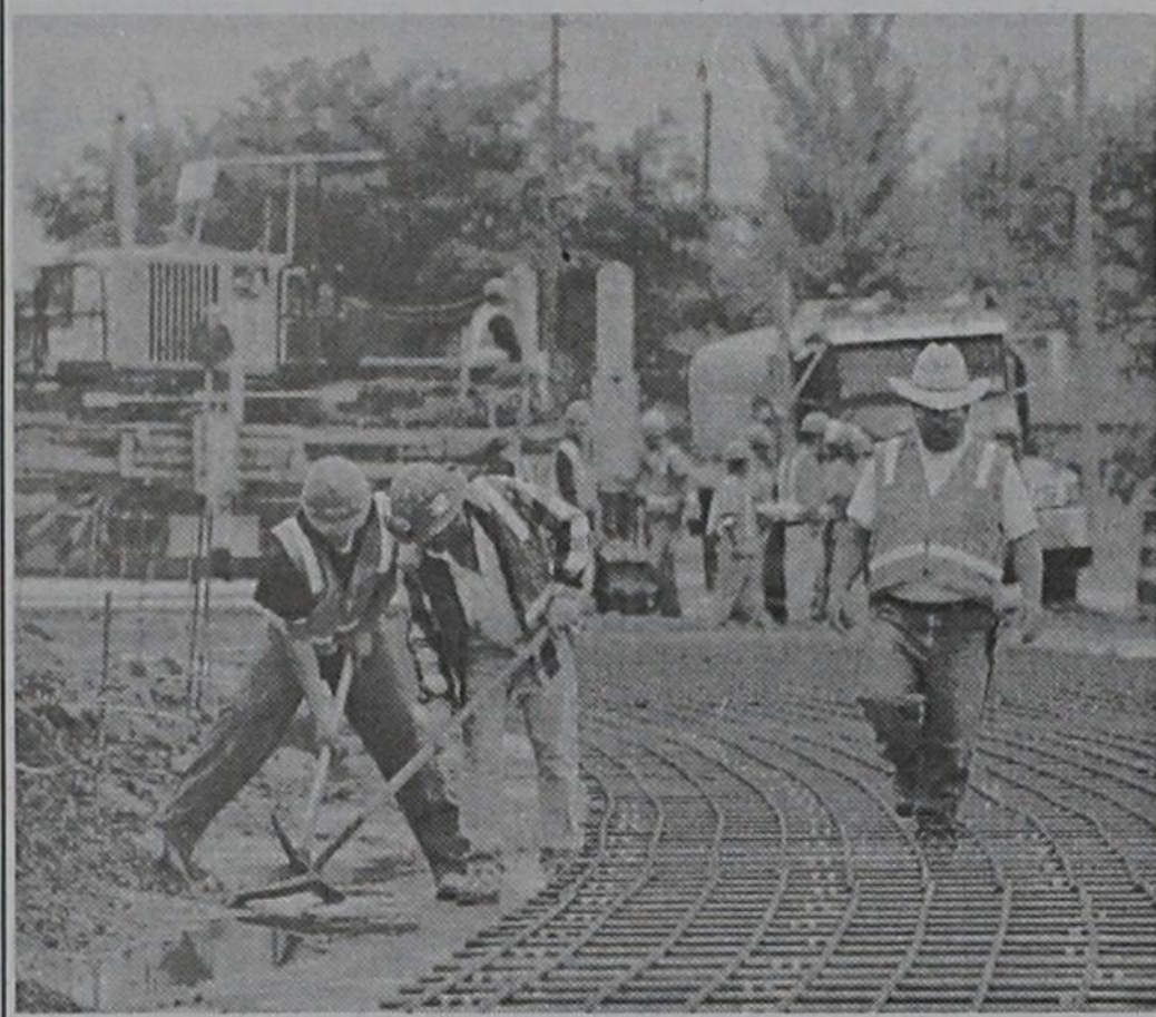
Granite Construction crews have been working long and late on the U.S. Hwy 84 project. Crews are pouring concrete along the west side of the roadway. (Photo by Tim Burnett)
