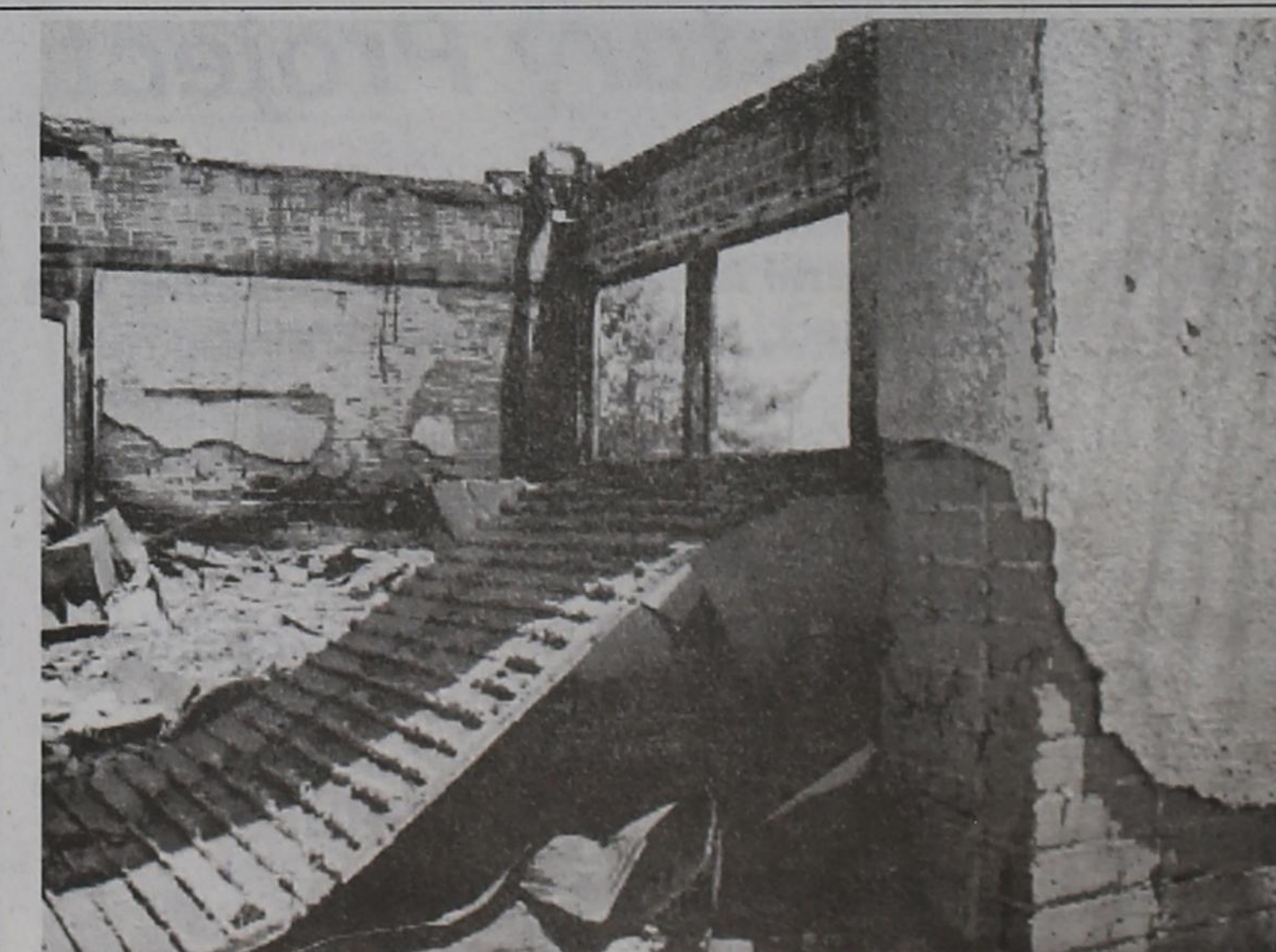
A fire last weekend at Justiceburg completely gutted the historic Justiceburg school house. Investigators are working to determine the cause of the blaze. (Photo by Tim Burnett)
