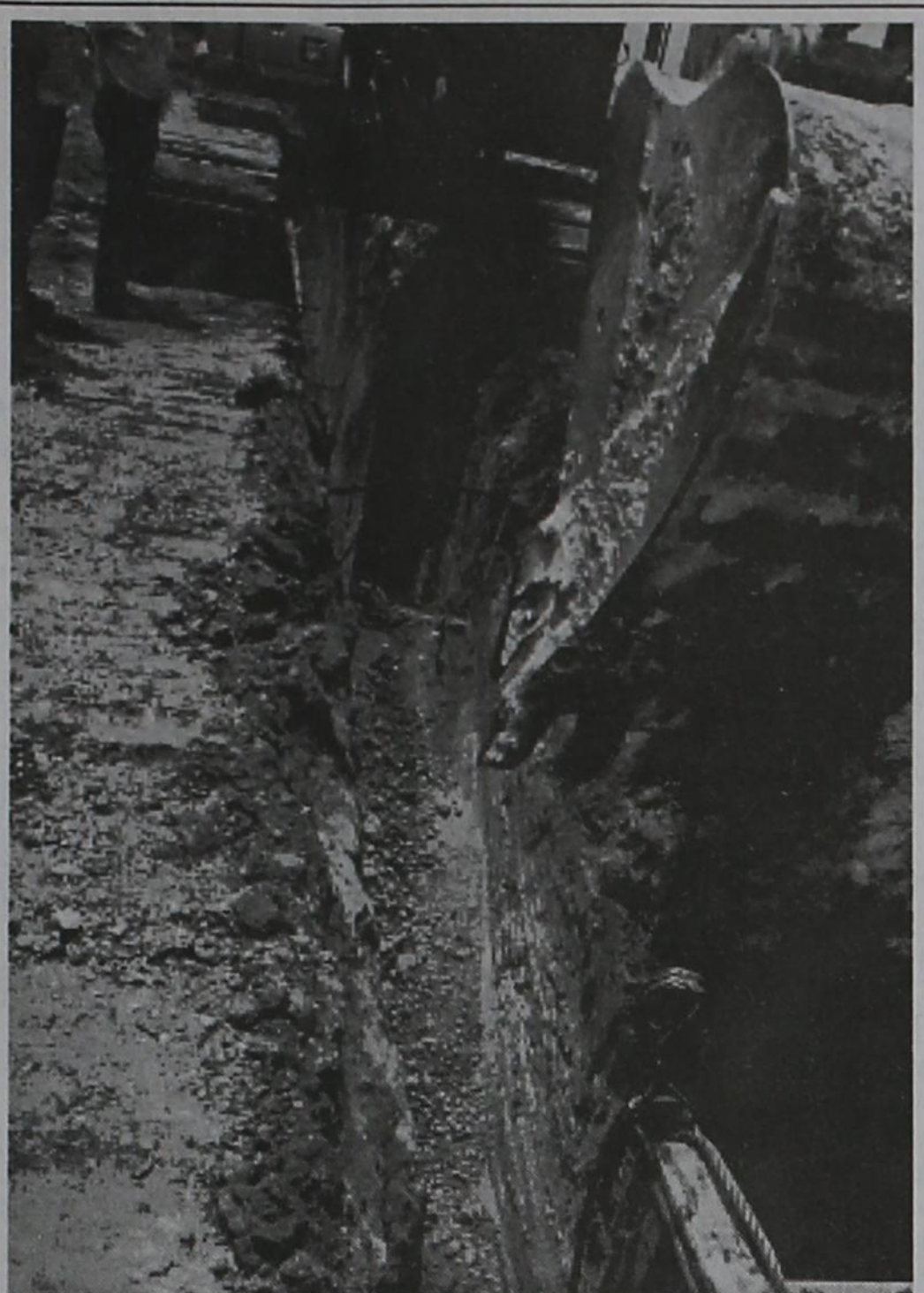
The final section of pipe was connected recently near Slaton as the Slaton-to-Post water pipeline project nears completion. The pipeline is being tested and storage tanks in Slaton and Post are being painted and getting final preparation requirements. Water is expected to flow through the pipeline within the next few weeks. When completed, the project will provide a backup water source for the City of Post.
