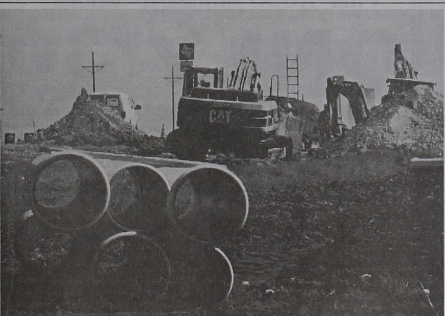
Construction on the pipeline between Post and Slaton is progressing on schedule. Engineers for the project expect the pipeline work to be completed by the end of July 2003. (Photo by Timothy W. Burnett)
