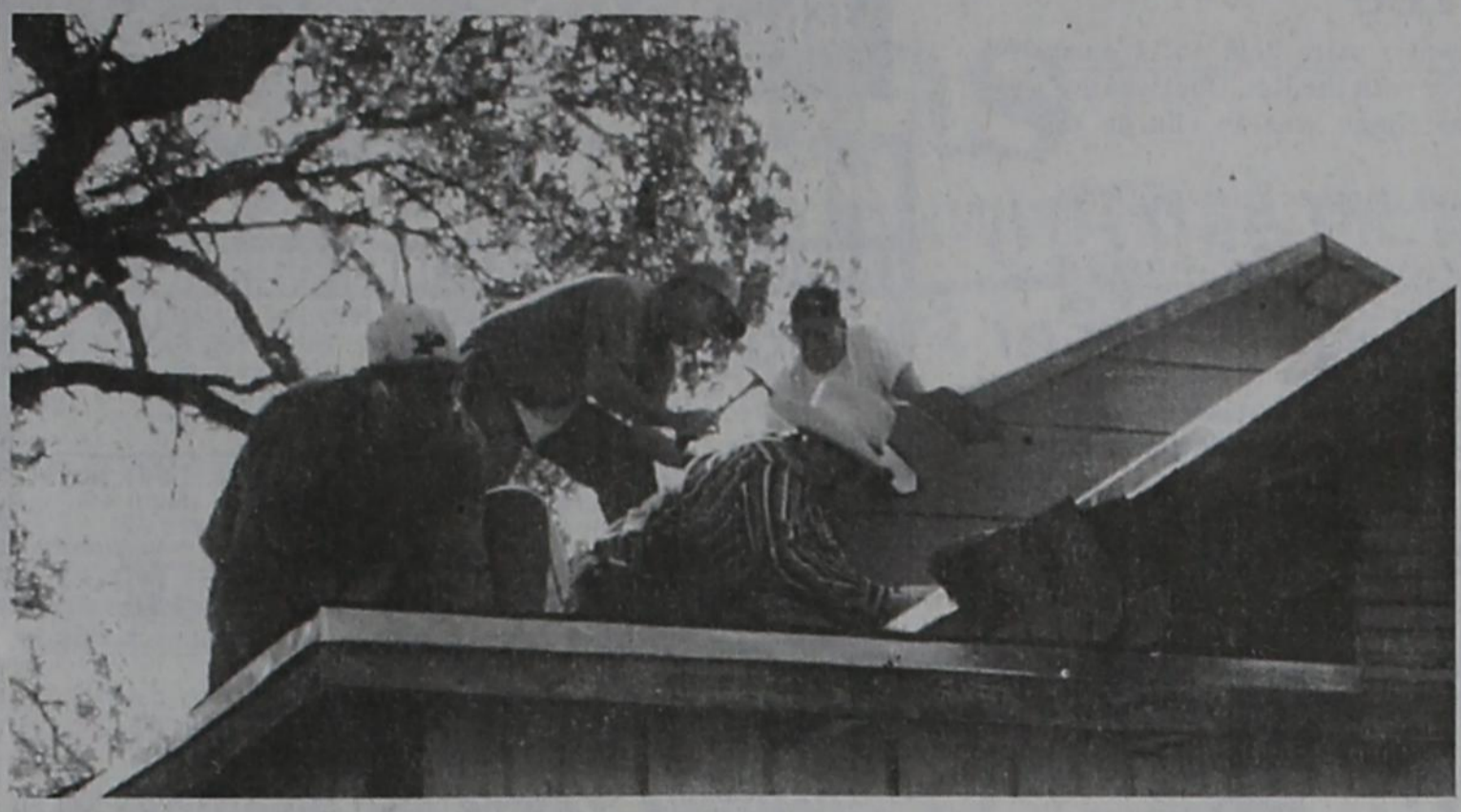
Backyard Missions volunteers put the finishing touches to a new roof in Post last month. Backyard Missions seeks volunteers, call Billie Williams at 495-2329 or Bryan Brownlow at the Post Middle School.
