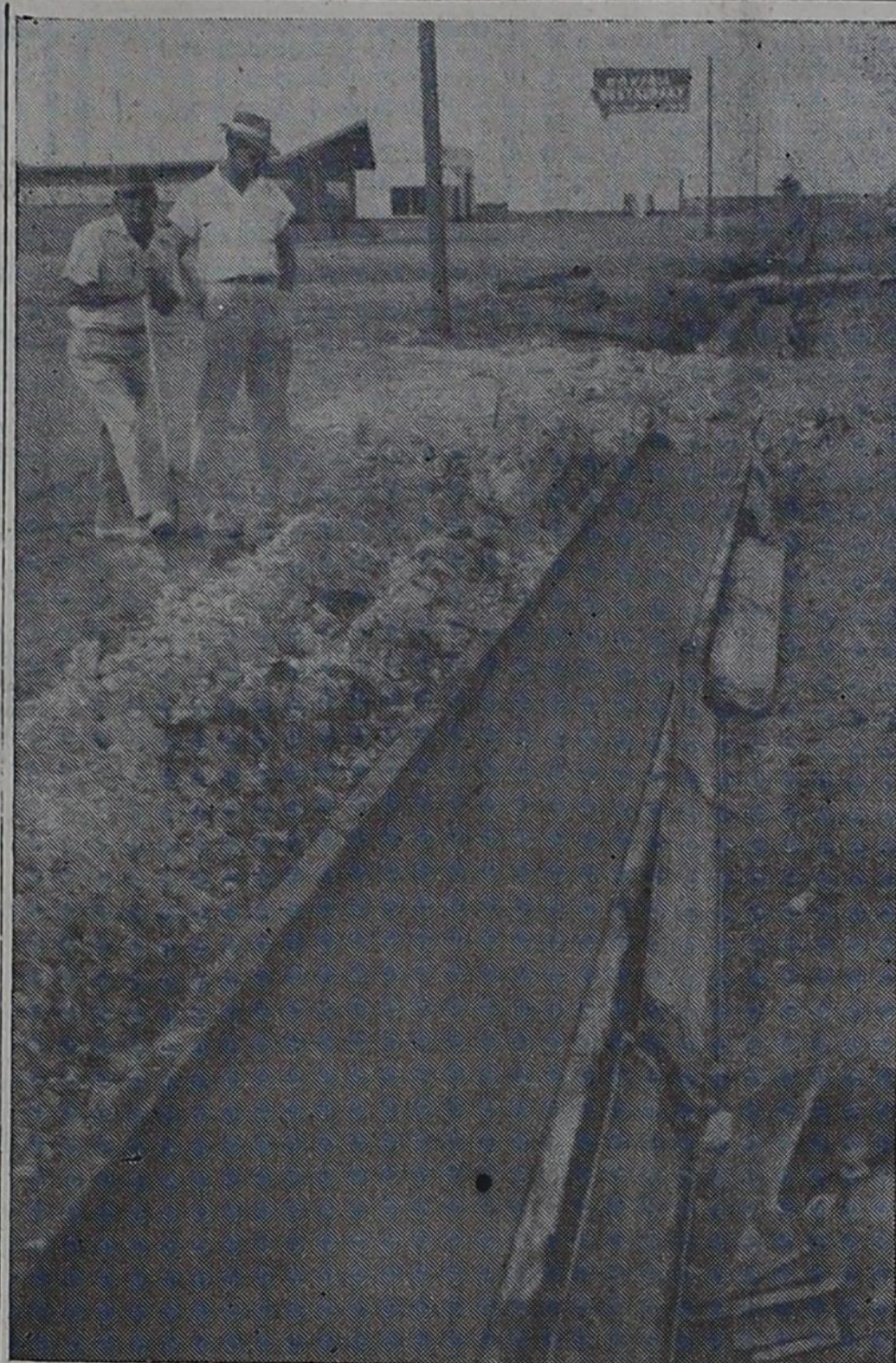
CURBS AND GUTTERS ARE GOING IN —Construction began last week on three blocks of curbs and gutters on Highway 60 in Bovina. In the above picture, Raymond Sudderth, with shovel, and Henry Minter look over the recently poured concrete. In the right hand corner of the picture is dirt that Sudderth has filled in so that motorists may drive to his Sands Motel. The motel is located to the left of the picture.
