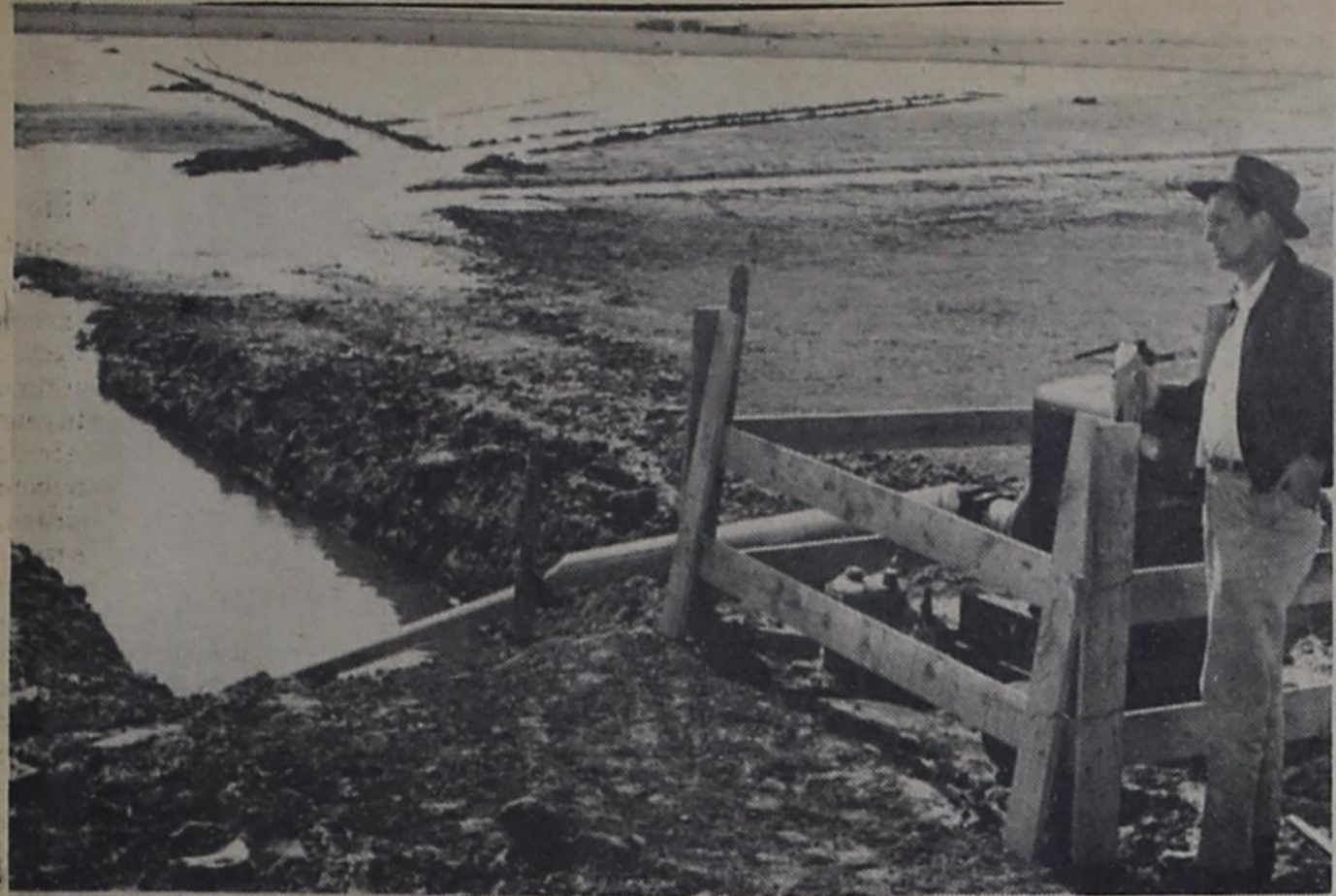
LAKE PUMP INSTALLATION... on Arthur Drake's farm southeast of Friona is one of the projects completed under the guidance of the county SCD office. Here, Bob Crozier, SCD representative, looks over the installation.
