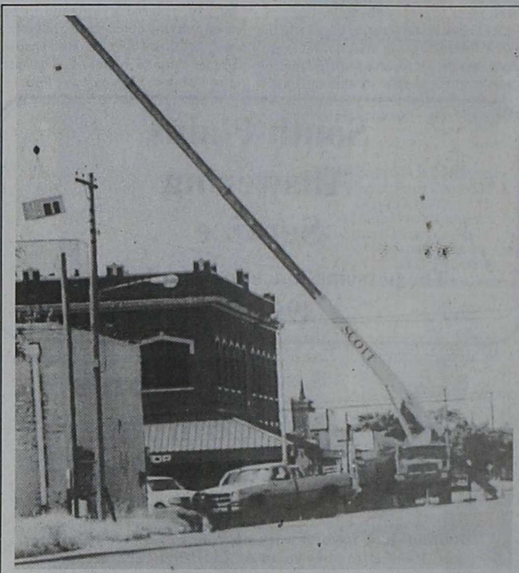
It took a special crane to mount an air conditioner on top of the McCrary building downtown last week. (Photo by Thomas Zachary)
