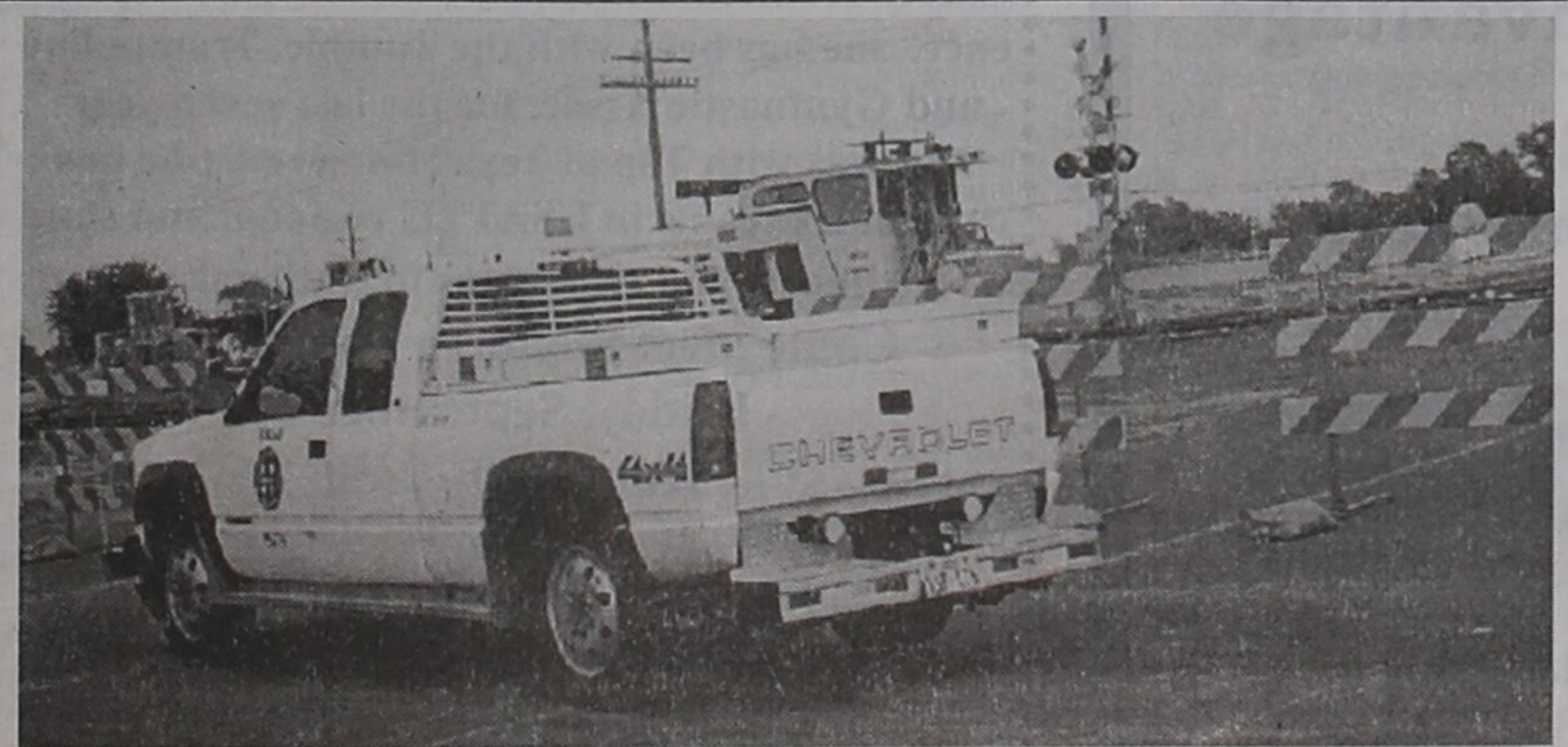
Burlington Northern and Santa Fe Railroad crews are finishing up repairs to the railroad crossing on East Main street. Detours were necessary for most of last week.
