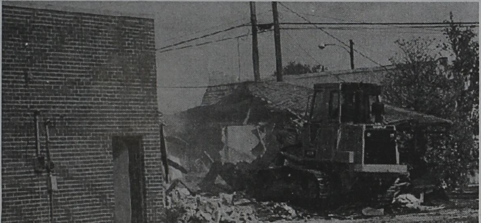
Demolition crews didn't take long to bring down Post landmark buildings last week in preparation for construction of the new McDonald's restaurant at the corner of U.S. Hwy 84 (Broadway) and Main Street.
