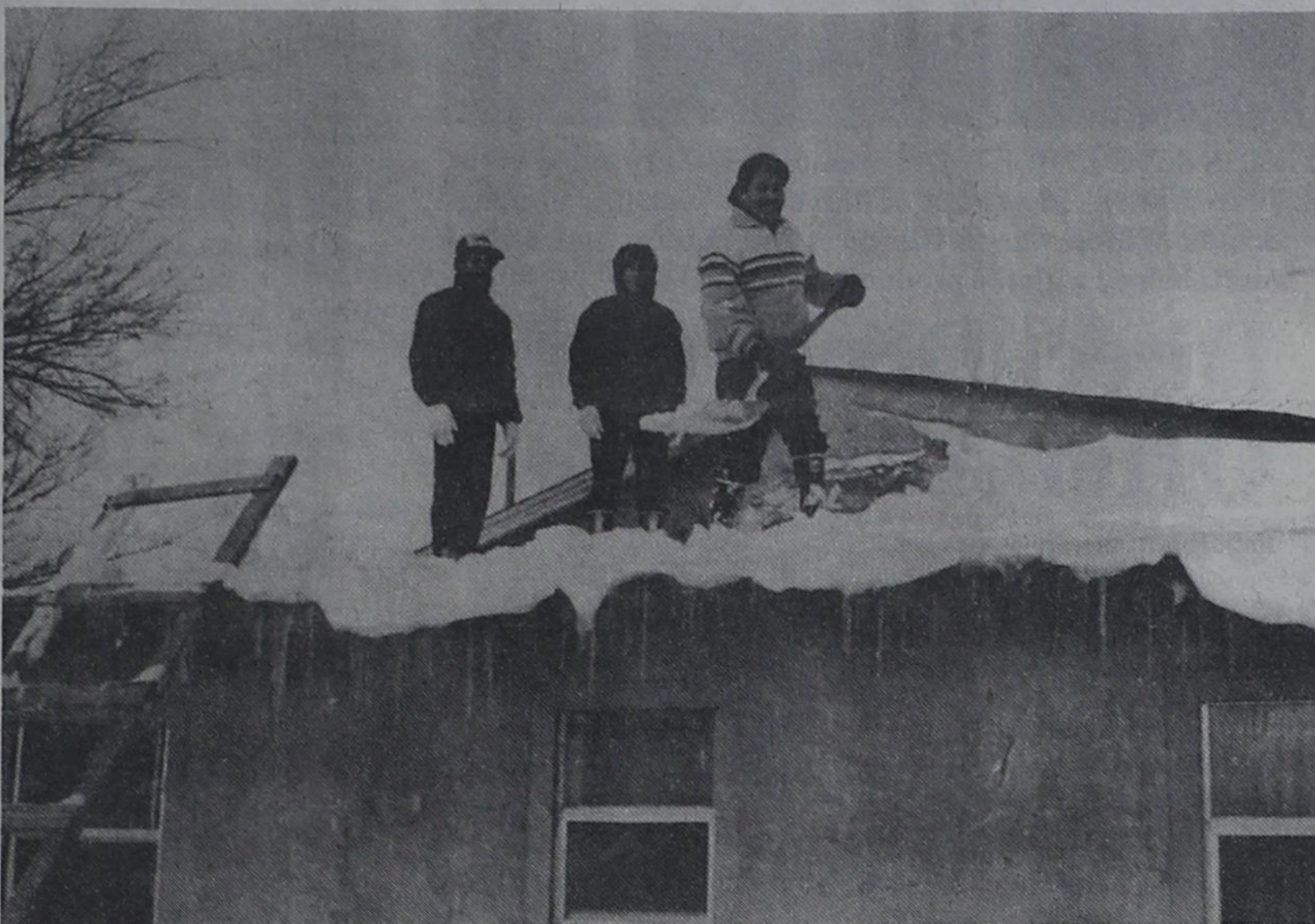
HIGH SHOVELERS... One of the unusual shovelling jobs Monday was at the Elizar residence on Seventh Street. Members of the family were afraid the extra snow might cause the roof to cave in, so they shoveled the snow off.
