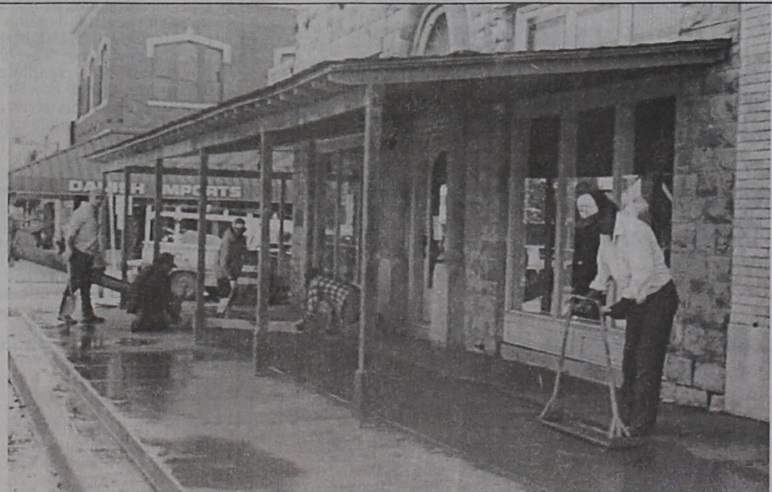
Sidewalk repairs continue downtown with work completed last Friday in front of the Algeria Art Center on East Main Street. Sidewalks and curbs are being replaced through a city contract, with individual property owners paying for their share of the work.
