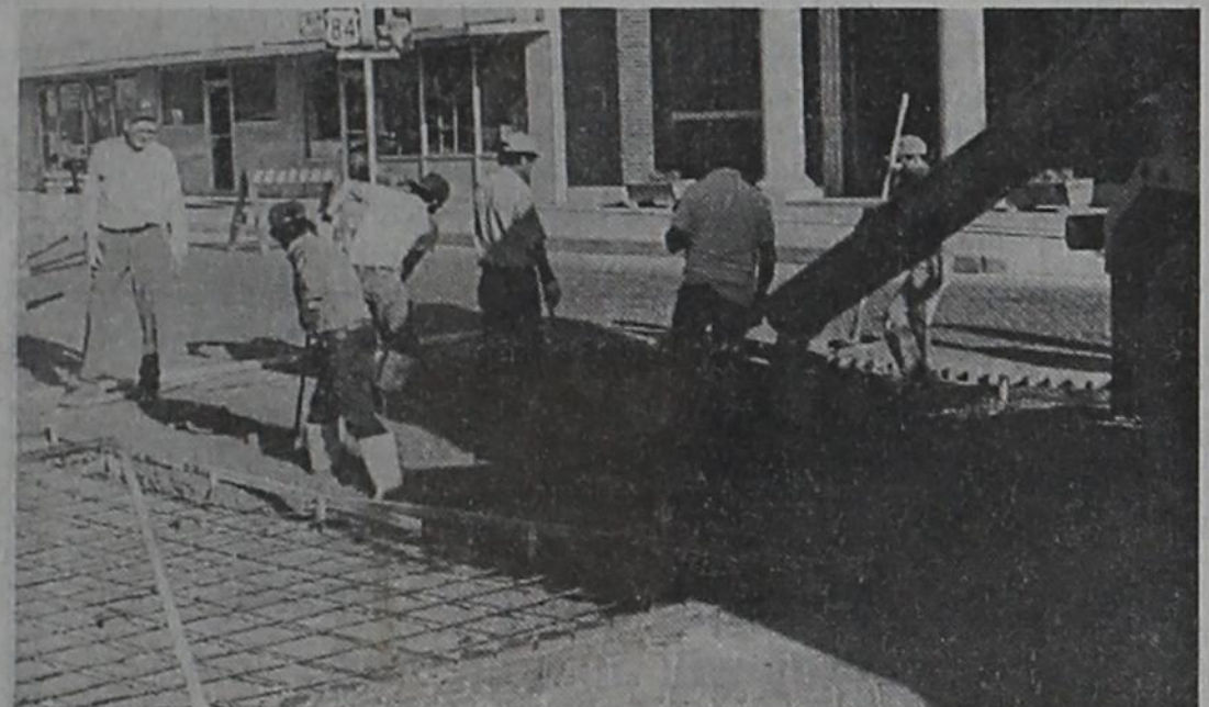
Concrete was poured last week at the intersection of East Main Street and Avenue H as Bo Jackson (left) supervises the work. The project is a joint effort by the City of Post and the Texas Department of Transportation.
