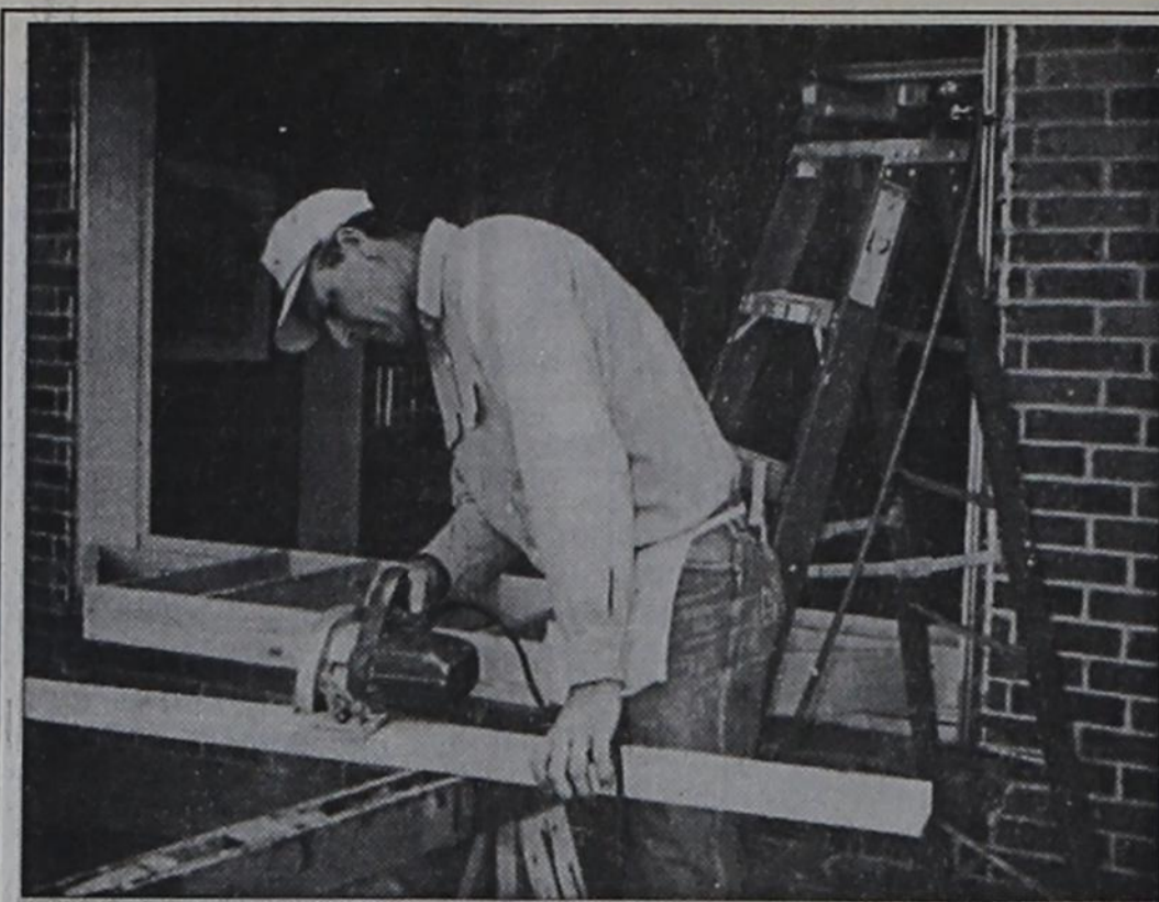
Larry Watson is repairing the window and trim at the Post Public Library. The window had been broken by vandalism and the trim was badly weathered.
