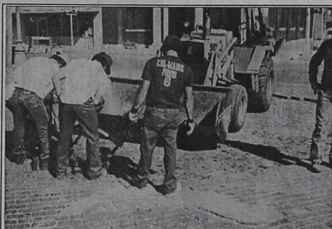
Construction began Monday morning to repair the intersections on East Main Street and Avenues H and I. The bricks are being removed and concrete will be poured at the intersections to prevent more damage to the bricks.
