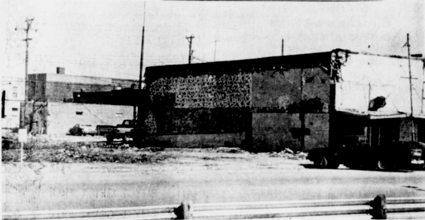
§ Mike Warren and Gregg Fisher next to their location on North 1st. city employees last week. [Staff photo] have completed the demolition The city library also was painted and clearance of two buildings at the east side of that block by
