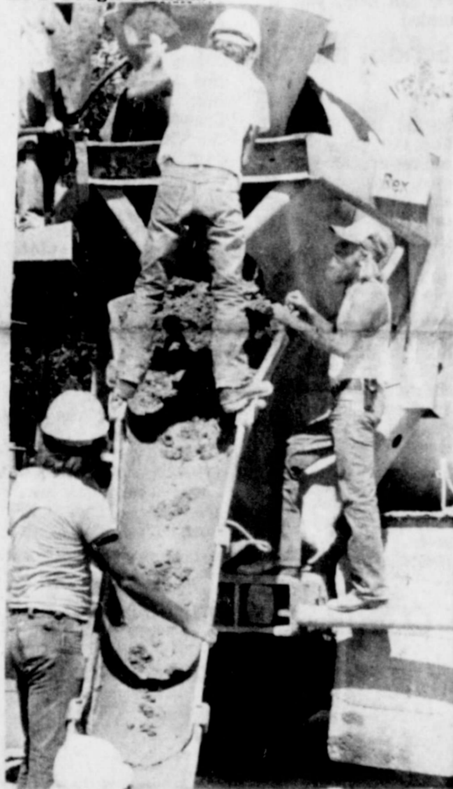
Workers started pouring concrete footings at Merkel High School last week. Workers should finish the footings this week. (Staff photo by Coy A. Richards)
