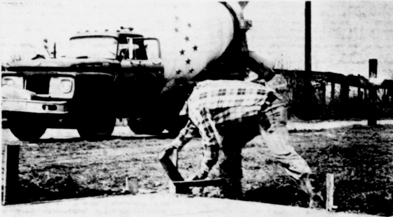
Ray De La Cruz puts some finishing touches on the foundation for a concession stand-rest room facility for the United Girls Softball League field. A work day had been scheduled for Saturday to
