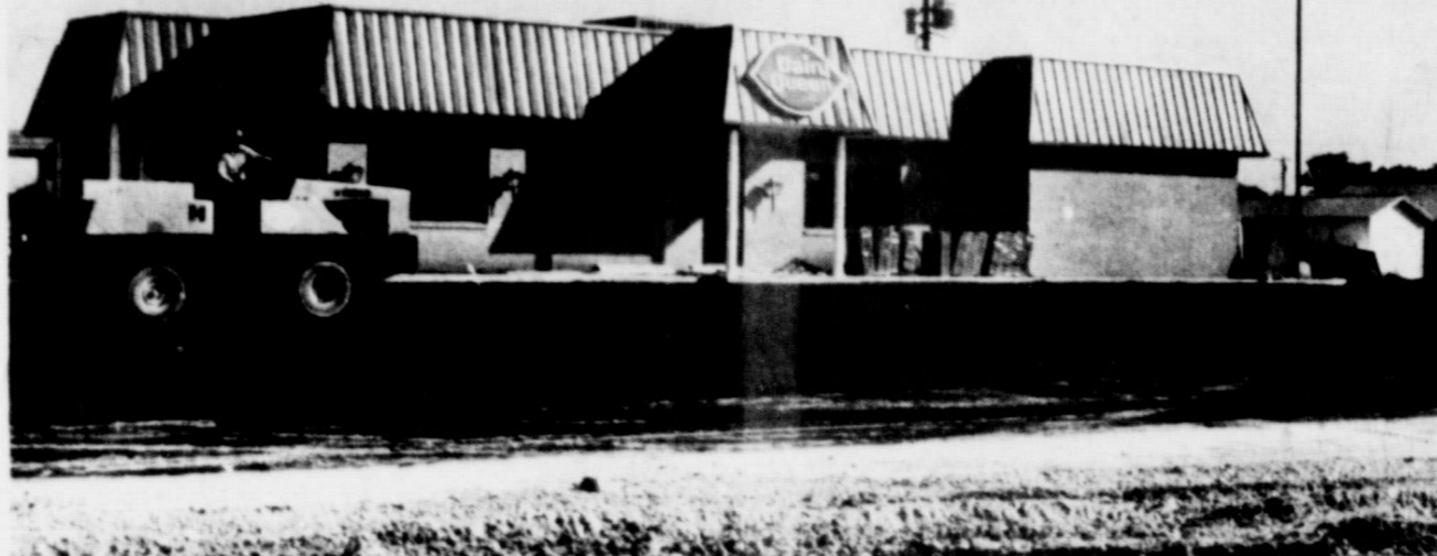
Workers finish the parking lot at the Merkel Dairy Queen last week. (Staff photo by Cloy A. Richards)
