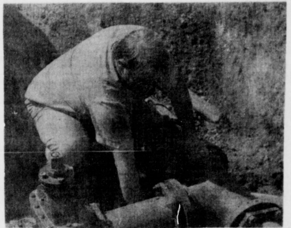
INSPECTING MAIN—Robert Harris, city employee, is shown inspecting the intersection of two water mains. The intersection was made in the early morning hours Monday and the new line will provide water for the Starr Nursing Home installation of automatic sprinklers which will further improve the fire-resistance of the home. J. A. Sadler, city coordinator, informed us that the water line was installed by the city at a nominal charge to the owners of the nursing home. The intersection is located west and one block north of Taylor Electric Cooperative.
