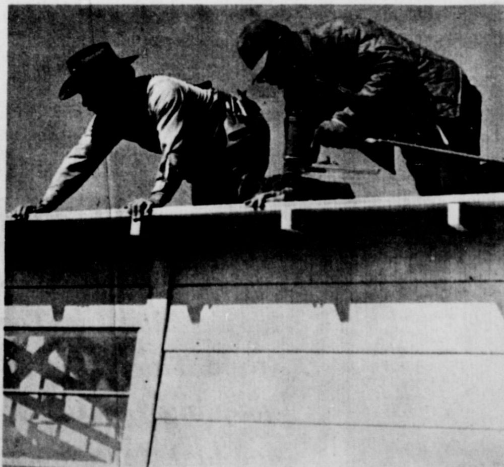
NEARING COMPLETION-The Bassett MFG. Co.'s "sales model" home was nearing completion late last week when this picture was taken. The modular home company is located in Industrial Park on I-20.
