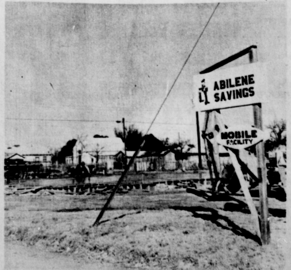
ANOTHER BUSINESS UNDER WAY-The new branch office of Abilene Savings which is being built in Merkel on Edwards Street across from Carson's Super Market is headed for a June completion date, said John Baker, superintendent at the site. A total of 120 working days have been allotted for the construction. Contractors are Rose and Son Construction, Inc., of Abilene. A mobile unit of the savings association visits Merkel twice weekly at the present time.
