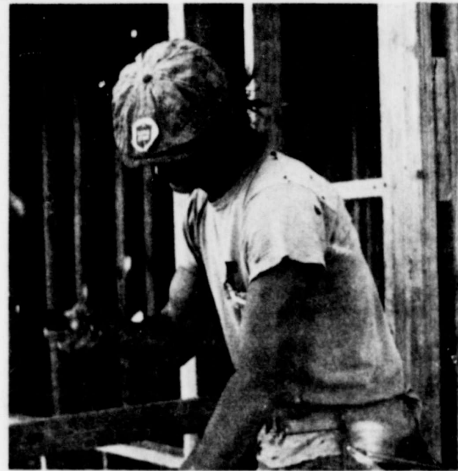
UNDER CONSTRUCTION-A construction worker hammers away at the construction site of the new apartment complex which is expected to be
