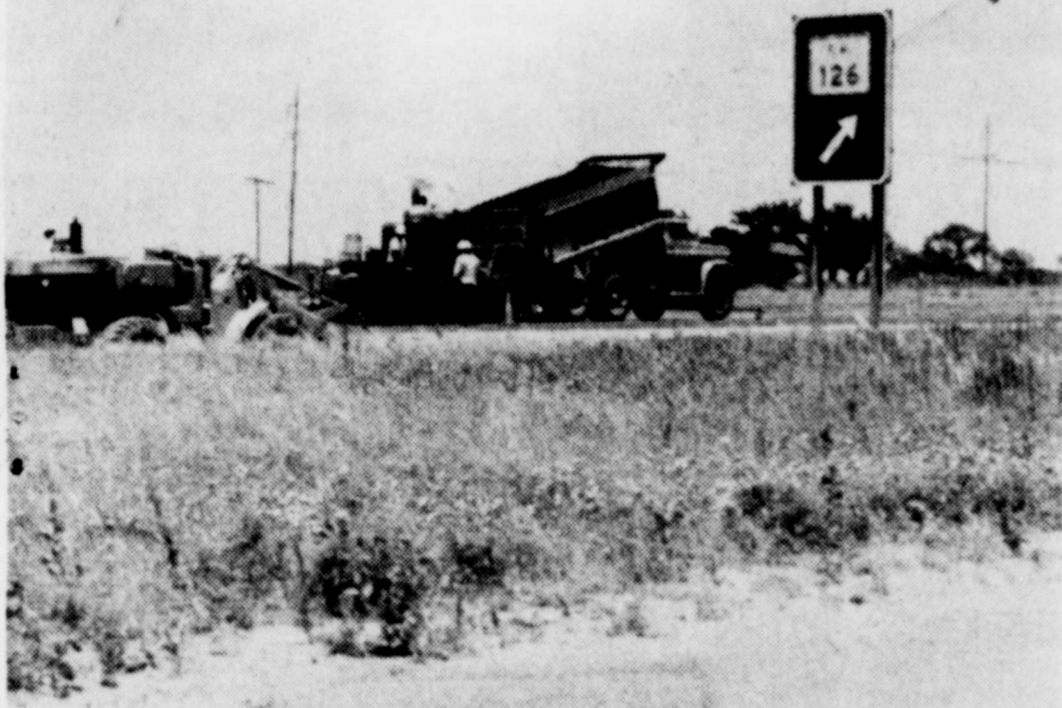
IT NEVER FAILS - Well summer is here and so are vacations. Unfortunately, invariably the Highway Department seems to always be busy tearing up and repairing the part of the highway that leads to your destination. Once in a while the tempers rise with the temperature, but let's face it, the fine highways that we have in Texas depend on these road crews keeping busy keeping them in shape.
