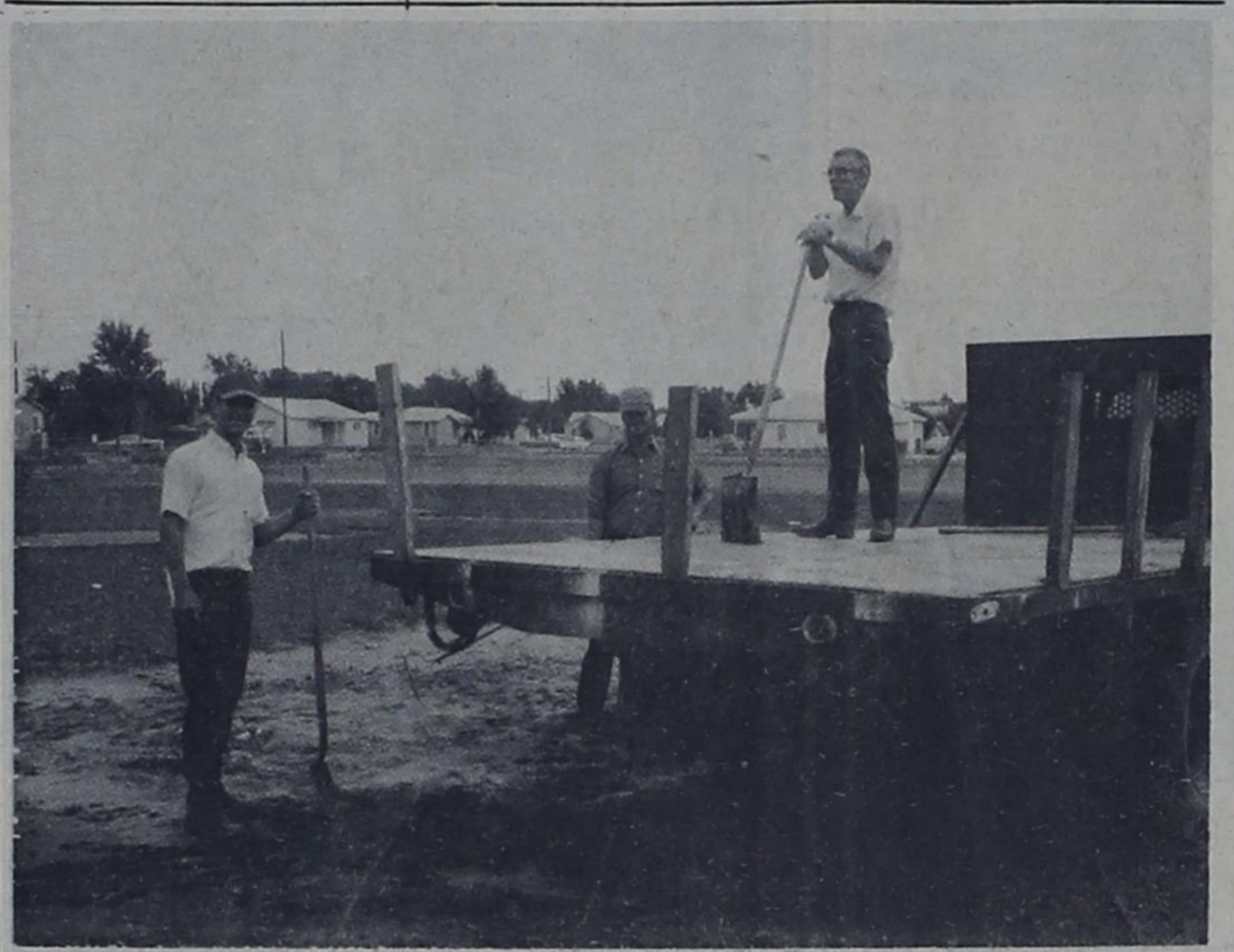
BALLFIELD IMPROVEMENT --- A broken waterline at the ball field here Monday caused base-paths and the homeplate area to be flooded with water. Sand was hauled in to absorb the excess moisture by this trio, left to right, Mac Glasscock, Kent Glasscock and Jim Russell. The field improvement was necessary so that Monday night's scheduled slow-pitch league softball game could be played. The five-week league is now just past the half-way mark.
