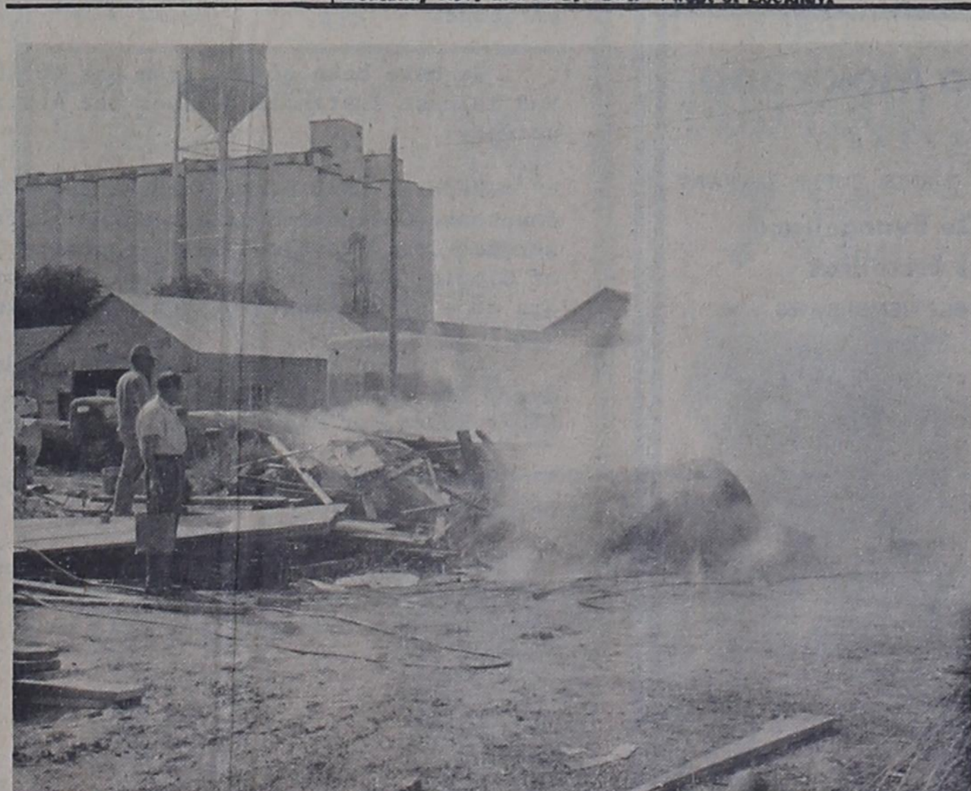
FIRE! -- A burning pile of scrap lumber at the new bank site Thursday was quickly brought under control by Bovina Volunteer Fire Department and construction Superintendent John Adlong. Wayne Spears is shown standing by with a water bucket in case things get out of hand.
