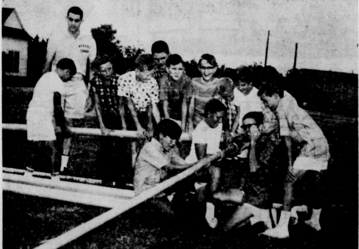
IRRIGATION CREW — Students of the Merkel Elementary School are busy connecting pipes to water the grounds between the Elementary and Primary schools. A beautification project began last year by the Merkel P-TA, grounds between the two schools are kept green with this process of watering. The P-TA raised funds for pumps and pipes which were installed last spring. In background is Elementary assistant coach, Eugene Boaz. (Staff Photo)
