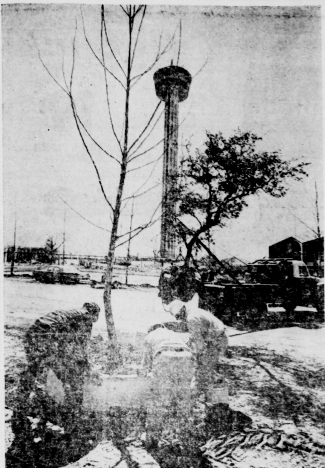
CHECKUP ON LANDSCAPING —HemisFair workmen are shown planting trees and grass early in April for the opening of the world's fair. Even though final touches have been made on tree planting, workmen keep constant check on growing trees.
