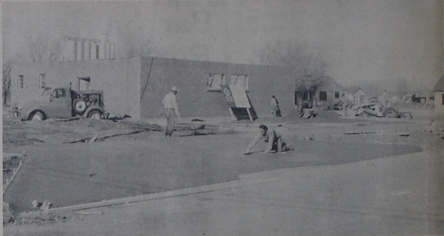
CONSTRUCTION ACTIVITY -- The site of Bovina's new post office has been a beehive of activity the past few days as construction on the new brick building continues. Concrete walks
