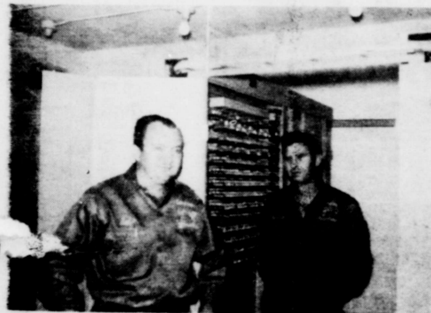
NOW YOU KNOW — Bob Huckaby, inside superintendent for Taylor Telephone Cooperative, Inc., and Derrell Farmer, outside superintendent, are shown inside one of the little houses that are central offices for Taylor Telephone's automatic dial system.
