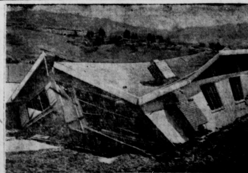
HOUSE OF CARDS . . . Undermined by severe rain storm, hundreds of homes in northern California were damaged like this one at El Sobrante.
