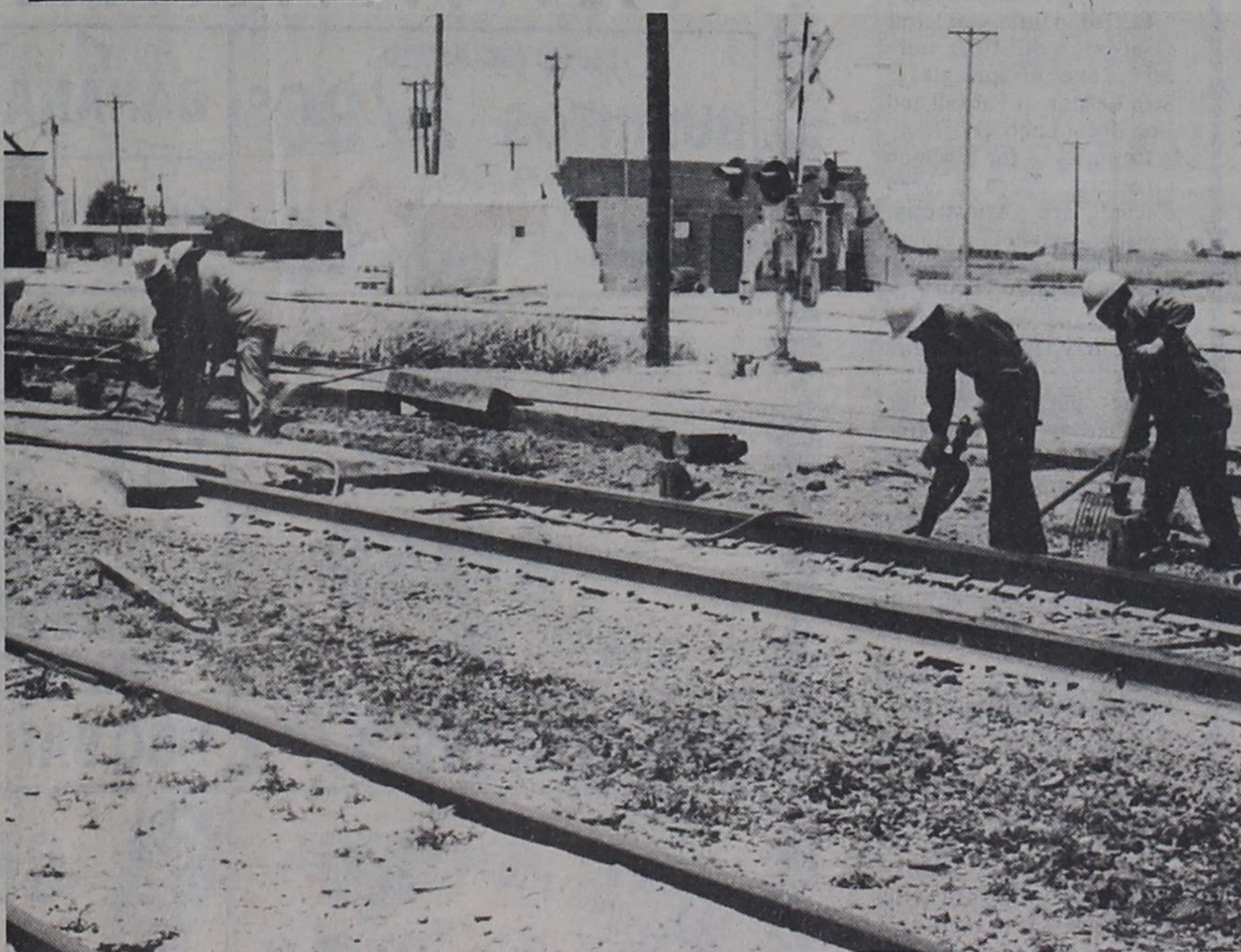
CROSSING WORK.... Employees of Santa Fe Railway have been reworking the railroad crossing on the east side of town this week. Motorists have been obliged to use the Third
