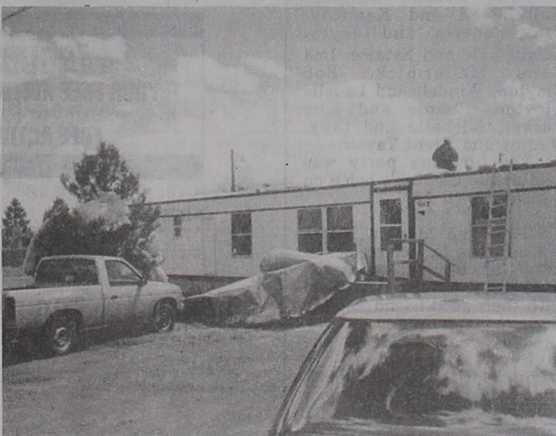
WIND DAMAGE... The Steelman property at the corner of Avenue I and Fourth Street suffered some major damage in the 55 to 60 mph winds which blew all day last Tuesday.
