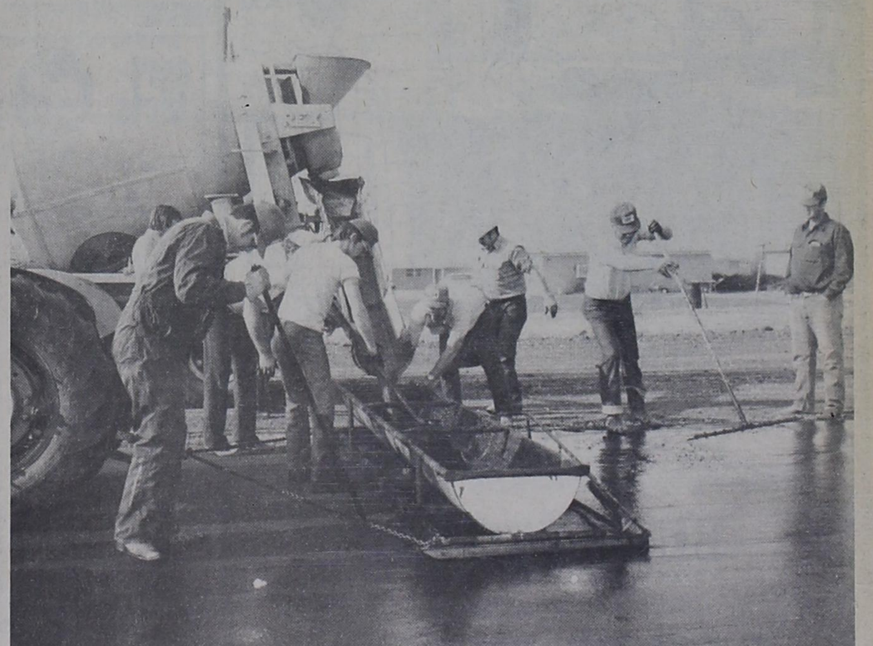
POURING SURFACE....A large number of Bovina men turned out Wednesday, Thursday and Saturday of last week to begin pouring the rubberized surface on the new track for Bovina Schools. However, the amount of material on hand was not
