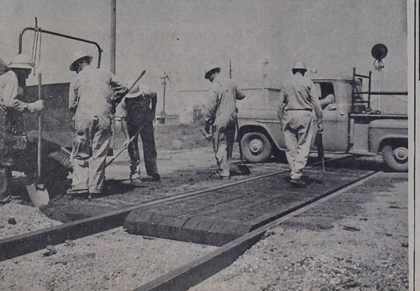
CROSSING REPAIR --Repair work on Third Street railroad crossing in Bovina Monday by this crew of Santa Fe workmen resulted in its being made safer and smoother for motorists. The men are shown putting the finishing touches on the job.
