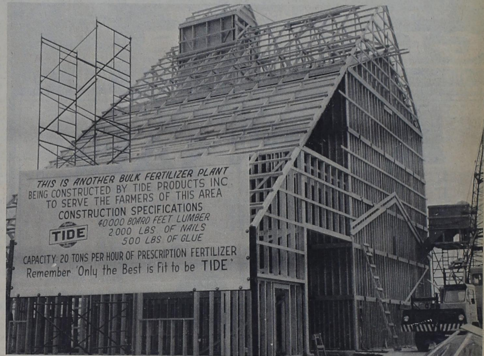
It takes a heap o' lumber to make a house a fertilizer plant, but 40,000 board feet did it in this large, unusually-shaped building under construction on Highway 60 near Farwell. It is for Tide Products of Edinburg, and will be one of five the company is building on the plains. Construction is expected to take another month.
