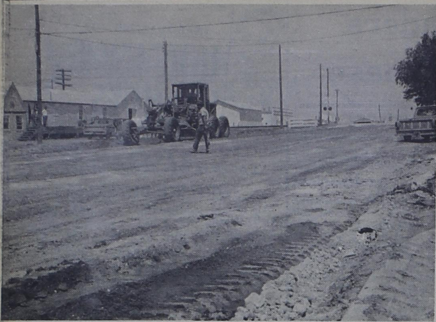
MORE STREET WORK -- This was the condition intersection of Third and Main Streets was in early this week as work on additional paving in Bovina continued. Traffic was not detoured around the intersection and resulted in confused and bump-shaken drivers.
