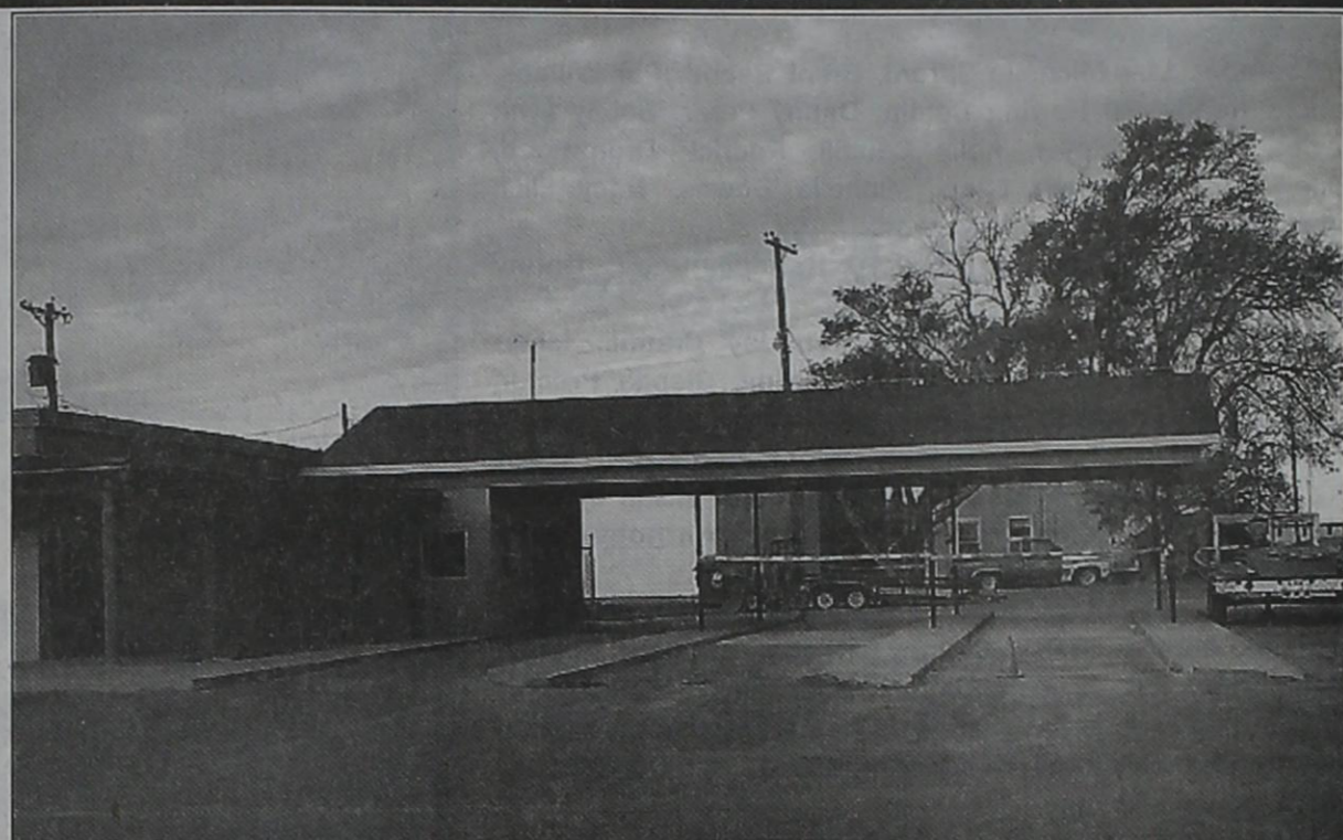
CONSTRUCTION continues on the drive thru lanes at the Friona Texas Federal Credit Union.
