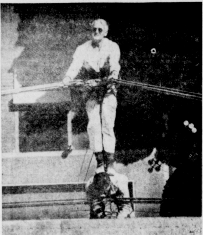
IT KEEPS HIM ON THE JOB—Here's an idea for keeping your workers on the job, boss. Suspended 300 feet above the ground, a stepladder at the University of California, Berkeley, plants his feet against the shoulders of his partner to help the lower man apply enough force to a drill he's using on the face of a big clock. The stepladders are repairing a faulty number on the clock's face.
