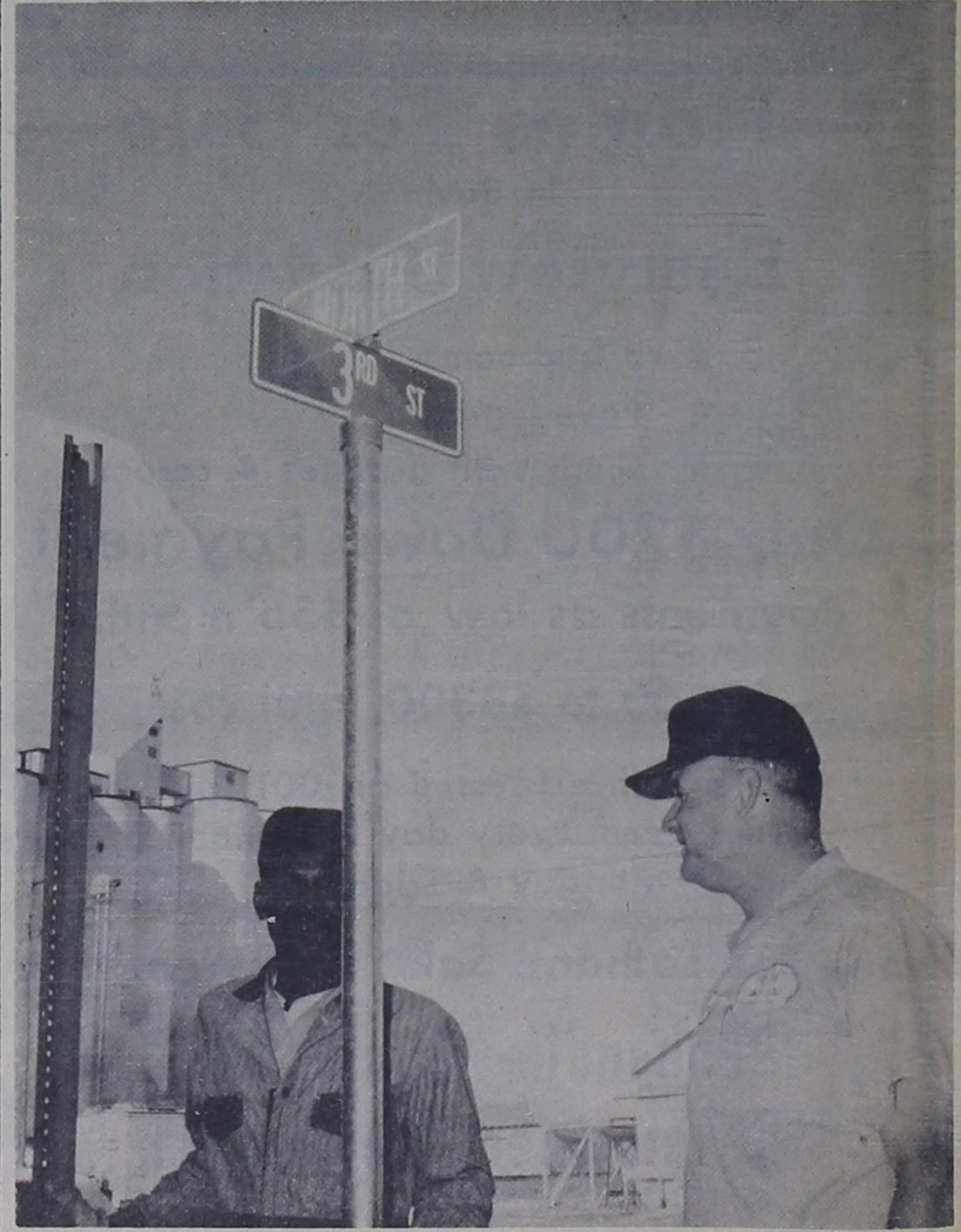
NEW STREET SIGNS --- Erecting new street signs in Bovina this week are Leon Clemons, left, and Darrell Reid of the city's staff. The signs are being put up on Bovina's main streets and are bright orange with white lettering. The metal posts holding the signs are being set in concrete.
