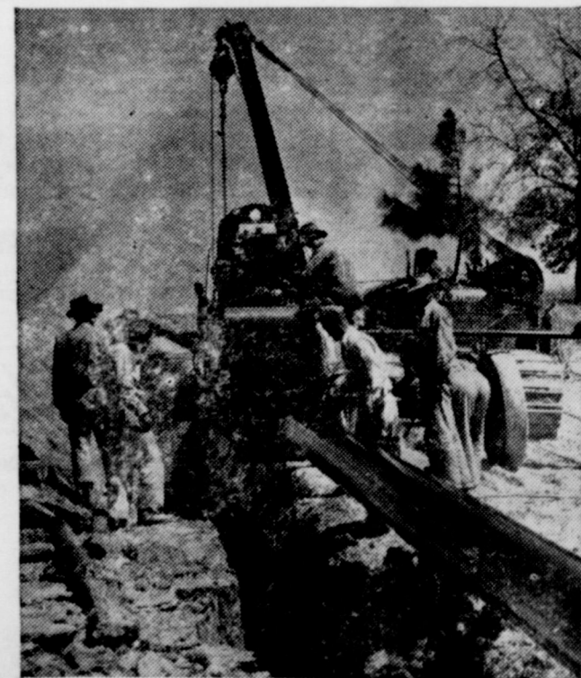
ONE OF SEVERAL NEW PIPELINES recently completed to keep gas service ahead of increasing demand. Since V-J Day, Lone Star has invested over $100 per customer in new facilities to assure each a dependable supply of gas. Yet for a year around average of less than 15¢ per day, you enjoy carefree heating, silent refrigeration, automatic cooking and abundant hot water supply using Lone Star Gas Service.
