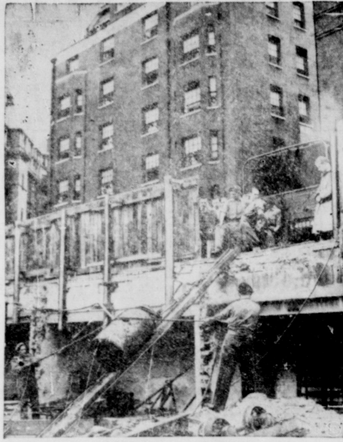
NINE YEARS LATER —Nurses and patients watch men of London's Bomb Disposal unit bring a 2500-pound bomb to the surface after removing the fuse. The bomb, one of thousands dropped by the Germans in '40's blitz, had lain underneath a partly demolished building until it was discovered . . . nine years after being dropped.
