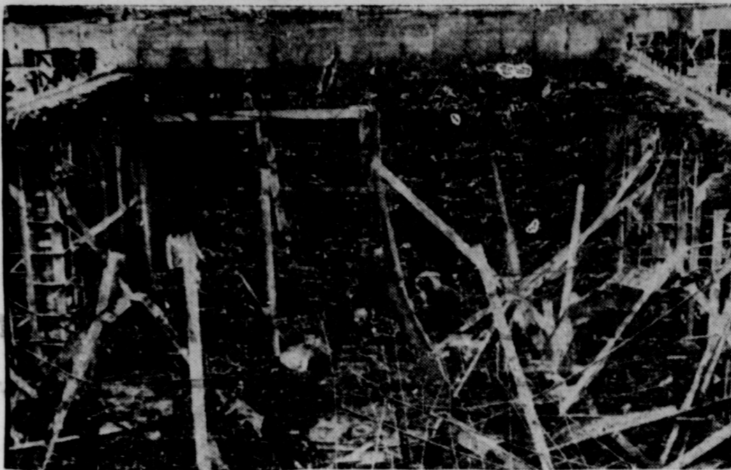
Eight workmen were injured when this concrete roof on a breezeway between two buildings at the Miamisburg, Ohio, Atomic Research Plant caved in. Two inspectors can be seen searching through the wreckage for clues as to the cause of the cave-in. (NEA Telephoto).
