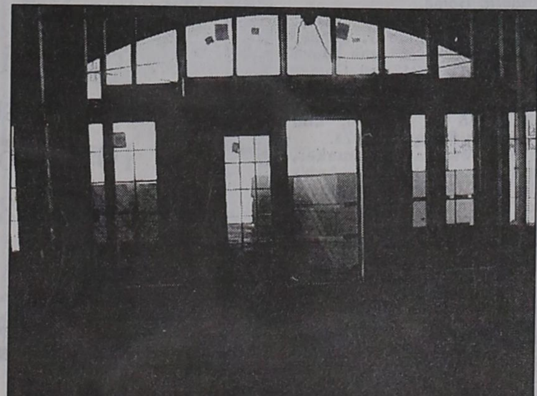
VIEWS among the construction at the new Heritage Estates addition to Prairie Acres. Left, looking out from the main door and
