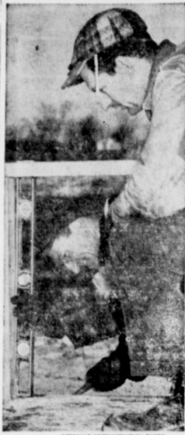
For a family of four facing eviction 15 days hence, a Barrington, Ill., family construction firm speeded a new home to completion with a day to spare. Handing the level is George Etton, World War I veteran, checking a back porch railing installed by his son, Earl, kneeling. Etton and his three World War II veteran sons started the business with the aid of a Veterans Administration-approved business loan.
