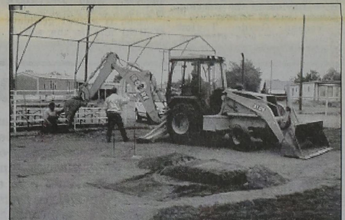
LITTLE LEAGUE PARK ---Just prior to the start of Little League season, the park has been rebuilt by Bovina city employees. New wood replaced rotting wood on the bleachers, the back stop was welded, new doors were built for the concession stand, new base paths were made for the new grass infield, and new bases were set in the ground. Plans to replace the lighting are also in the works.
