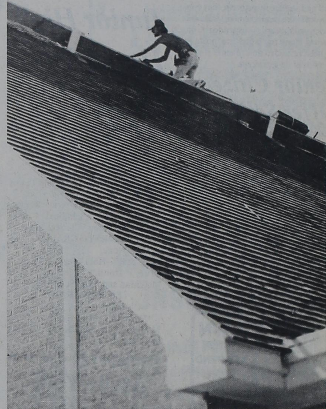
HIGH OCCUPATION....A workman has been busy this week putting a new roof on the First United Methodist Church
