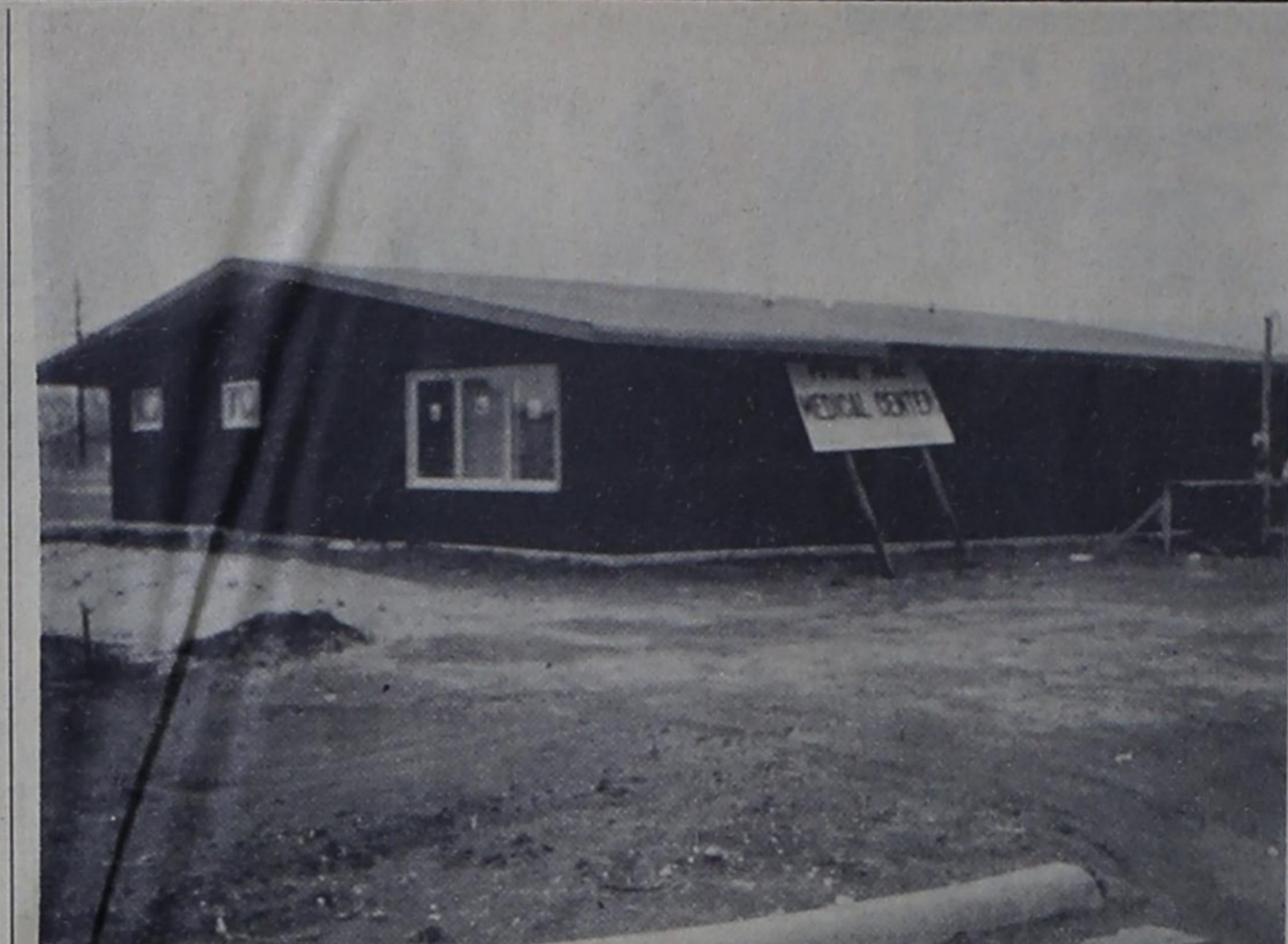
WALLS UP -- Progress was being made on construction of Bovina Medical Center, last week and since that time brick-laying has been about half completed. Work was interrupted Monday by snow. J. E. Sherrill, contractor, says the building should be completed by April 1.
