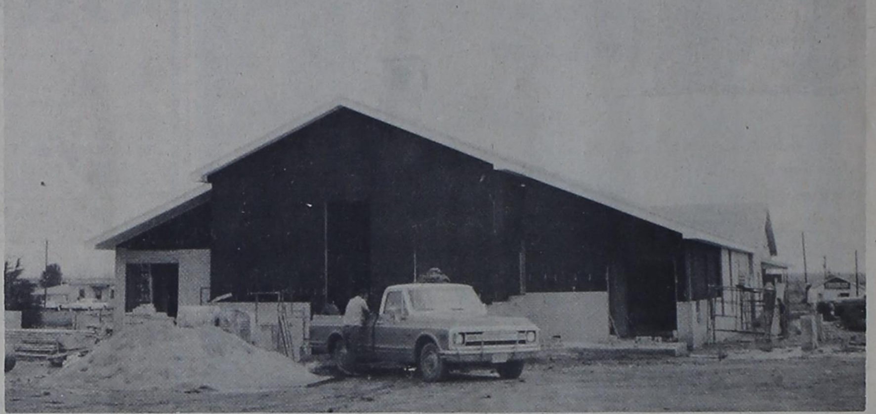
NEW CHURCH FOR ST. ANN'S --- Construction is in the final stages on the $65,000 sanctuary of St. Ann's Catholic Church on Third Street. The building is slated for occupancy early this fall. Ground-breaking ceremonies were conducted Sunday, May 16, with Bishop Lawrence M. DeFalco of Amarillo in charge of the ceremony. Franklin P. Bottoms, of Amarillo, contractor for the project, began pouring the foundation in the
